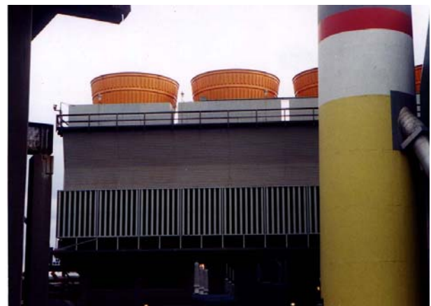
Hartford Cooling Tower: Hartford, CT
